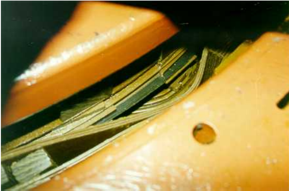
Top view on the common winding buckling in 200 MVA autotransformer Figure 8
